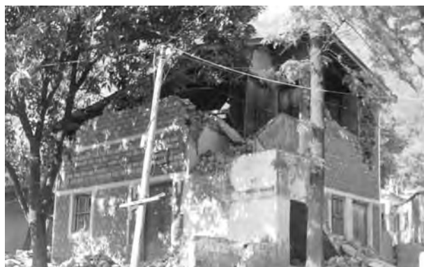
Figure 7.1 : A Damaged Building Due to an Earthquake
