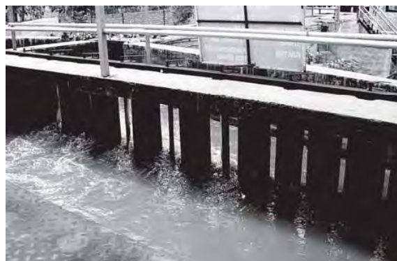
Fig.18.4 Grit and sand removal tank
