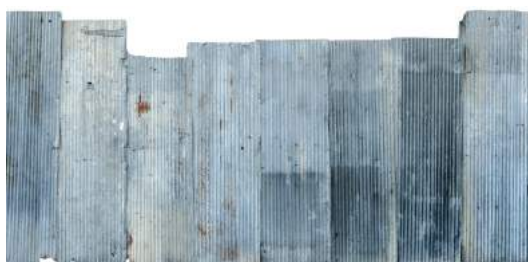
Fig 5.7 Damaged iron sheets
