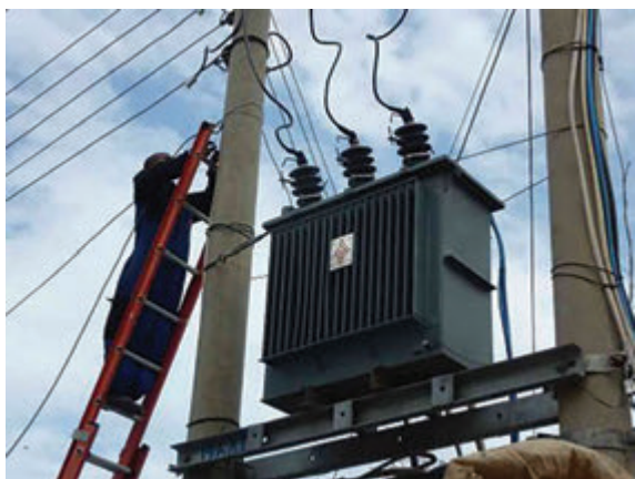
Figure 4.37(b) Roadside transformer
