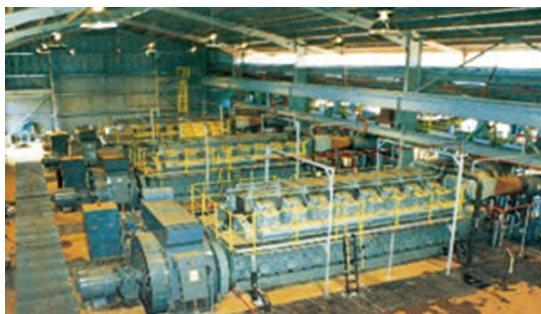
Diesel Power Plant (Chennai)
