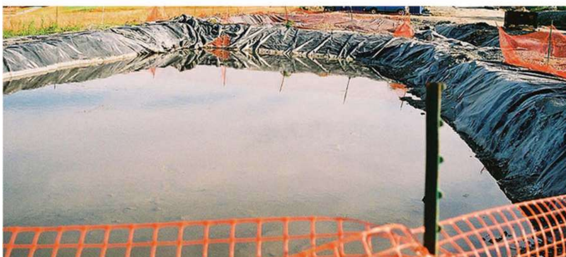
Silpaulin water storage tank
