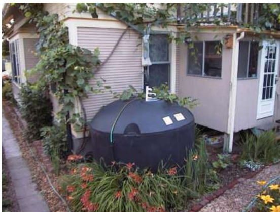
Rain water storage tank
