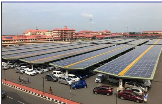
The Solar Power Plant at the International Airport, Nedumbassery. The Power Plant takes care of the complete energy needs of the airport and the excess energy is given to KSEB. It received the Champion of Earth Prize – 2018 instituted by the United Nations for its use of Green Energy.
